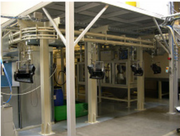
Flocking plant: general view
